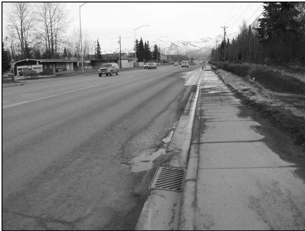
Photo 2.13: 7.5 year old SMA with AC-5 with +0.75-in ruts - Anchorage
