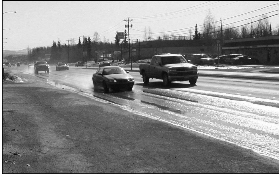
Photo 2.12: 10.5 year old SMA with AC-5 overlay with 1-in ruts – Anchorage
