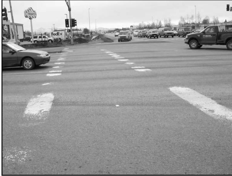
Photo 2.2: Anchorage Type I at intersection of Tudor Road and C Street, placed in 1991
