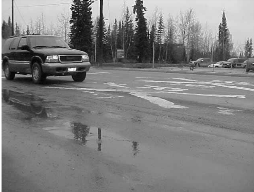
Photo 2.8: Pavement Rutting in Fairbanks – 12-year old pavement
