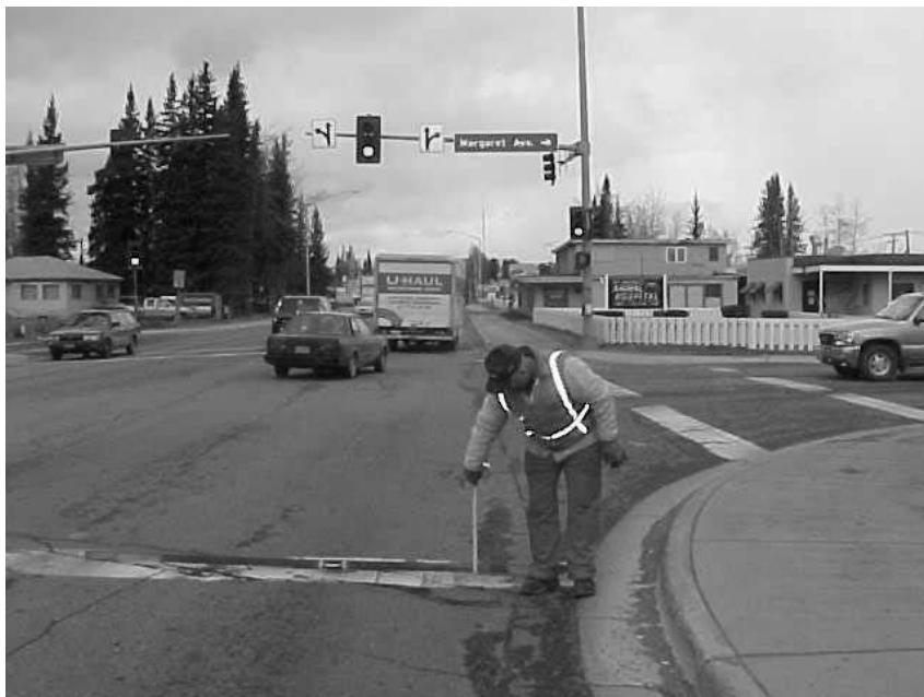
Photo 2.9: Pavement Rutting in Fairbanks – 18-year old pavement
