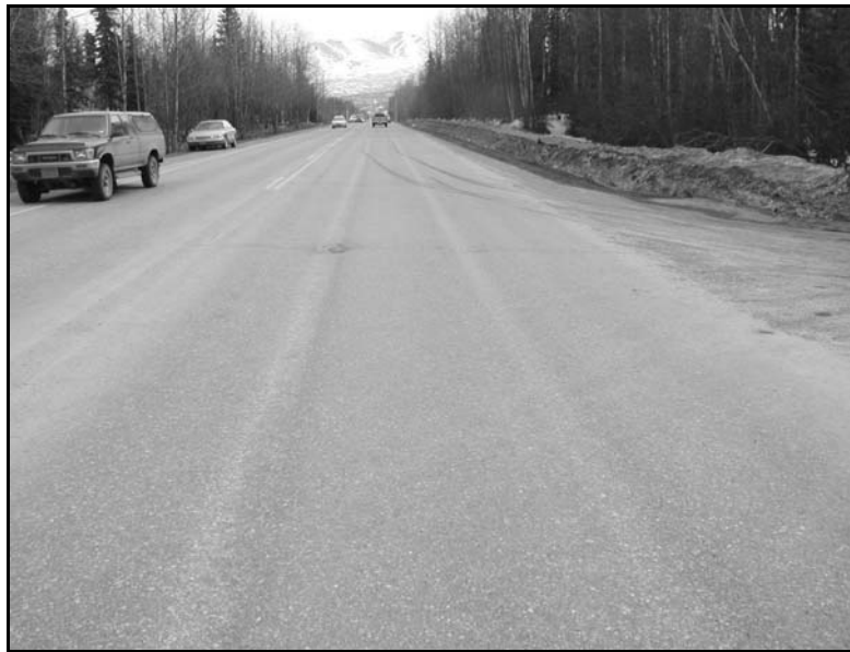
Photo 2.6: Anchorage, Type III Maintenance overlay, 3.5-years old
