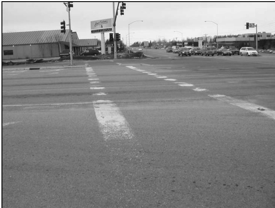
Photo 2.16: SMA with PG58-28, 4-year old mix in Anchorage starting to rut/wear
