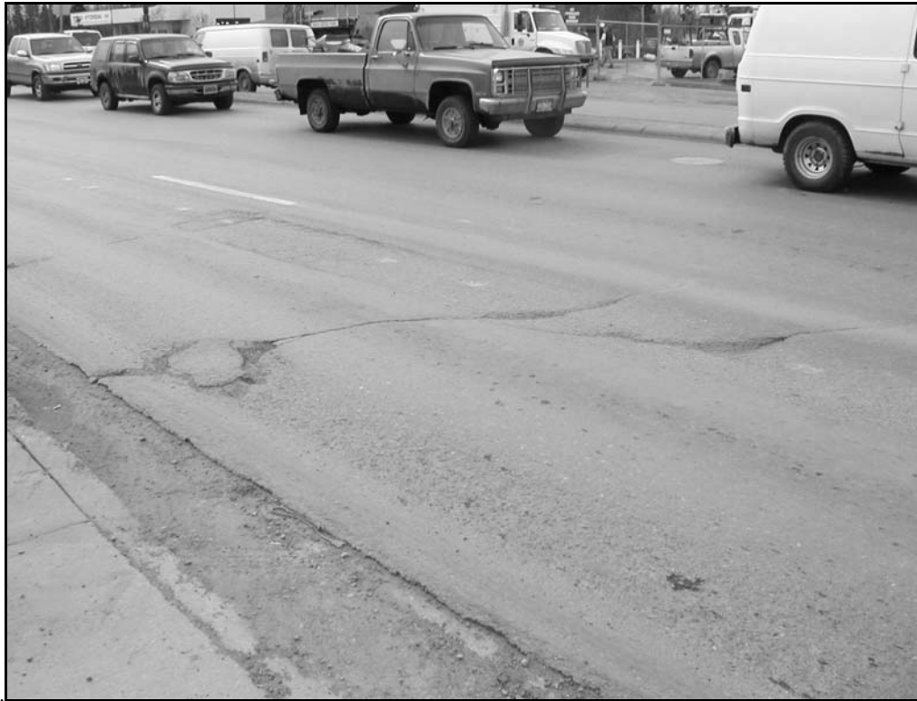
Photo 2.3: Anchorage Asphalt Concrete Type II mix placed in 1994 with nearly 2-in ruts
