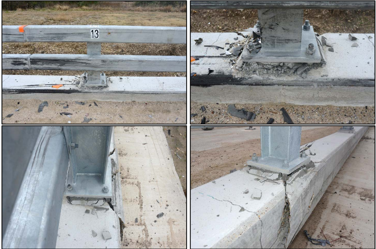
Figure 7.4. Damage at Post 13 after Test No. 608331-01-3.
