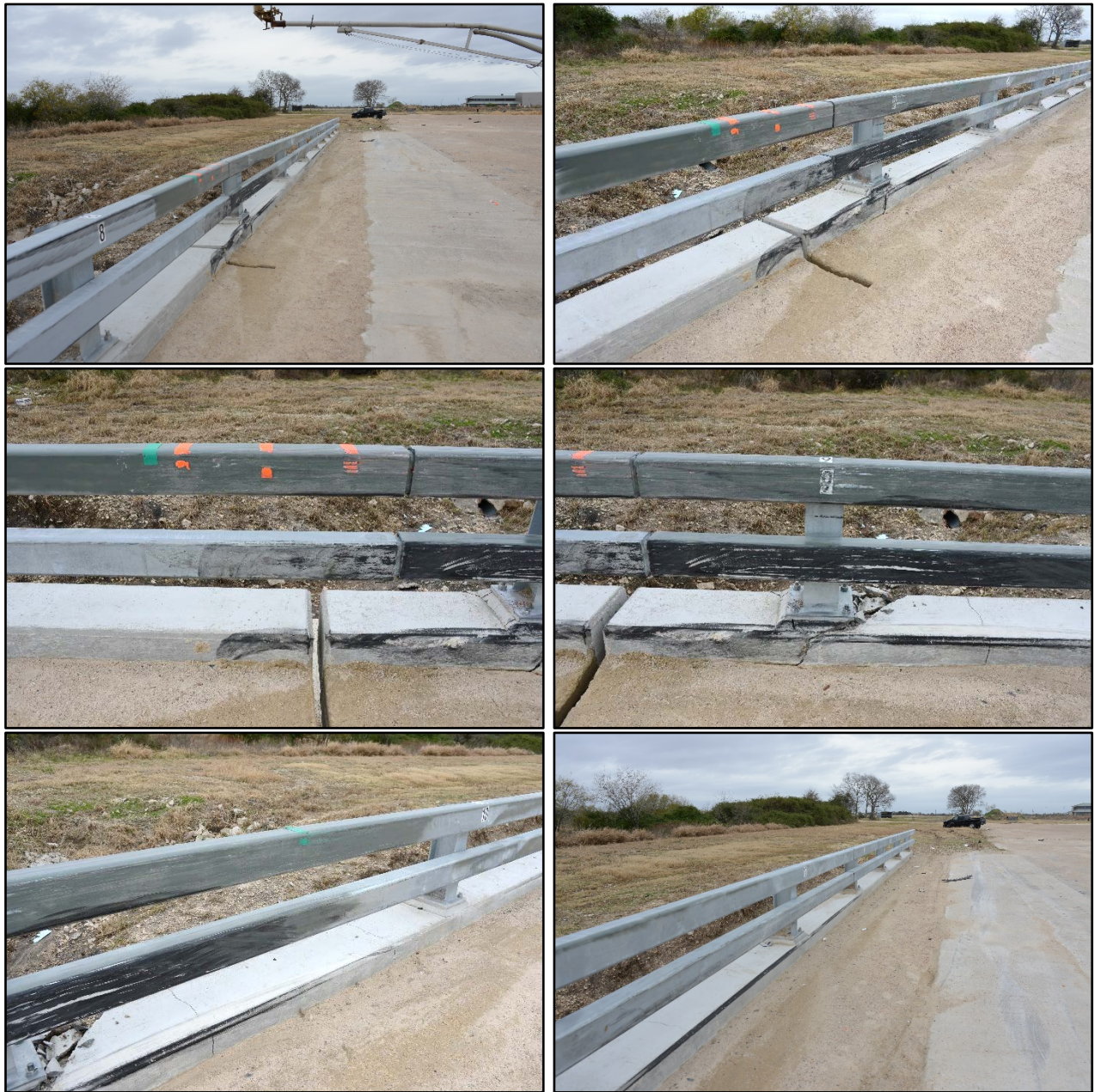
Figure 6.3. 2019 MASH 2-Tube Bridge Rail after Test No. 608331-01-2.
