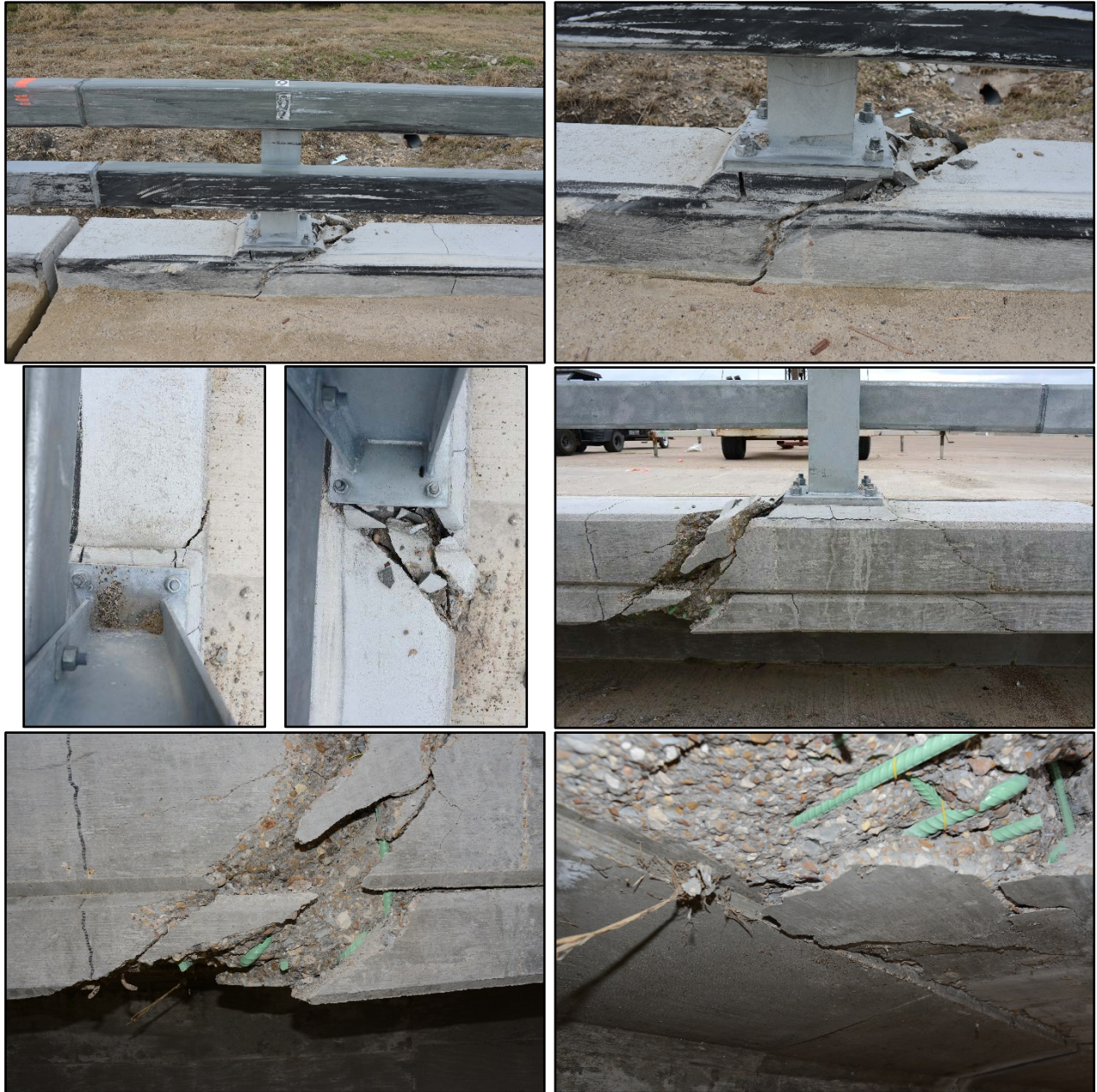
Figure 6.4. Damage at Post 9 after Test No. 608331-01-2.
