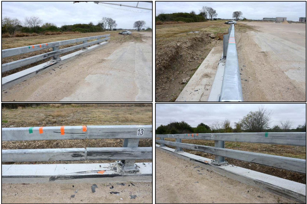
Figure 7.3. 2019 MASH 2-Tube Bridge Rail after Test No. 608331-01-3.
